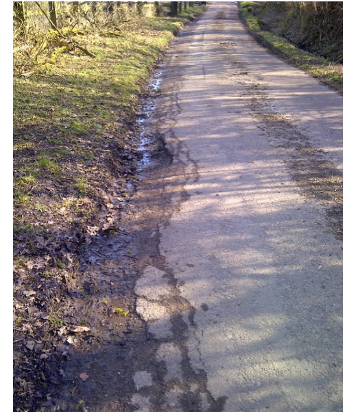
A typical fit for purpose rural unclassified road with some edge deterioration, over-riding, detritus and the occasional non-running lane pothole defect.
